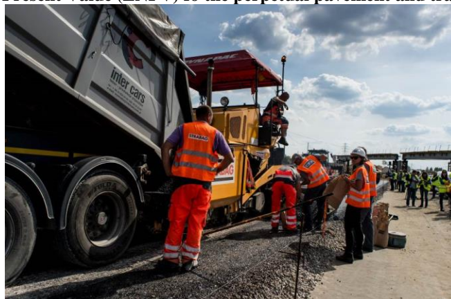
Figure 9: Construction of trial section of anti-fatigue course using special PMB binder, September 2014?
