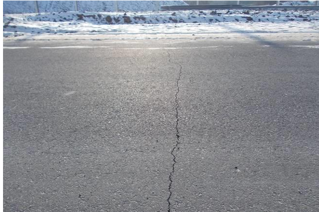
Figure 4: Low temperature cracking on unfinished pavement surface with high stiffness modulus courses with bitumen 20/30 during winter 2012
