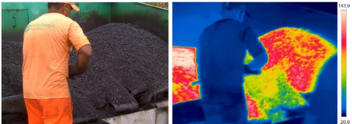
Figure 1: Thermographic camera image picturing the handling of asphalt which temperature scale is in Celsius.
