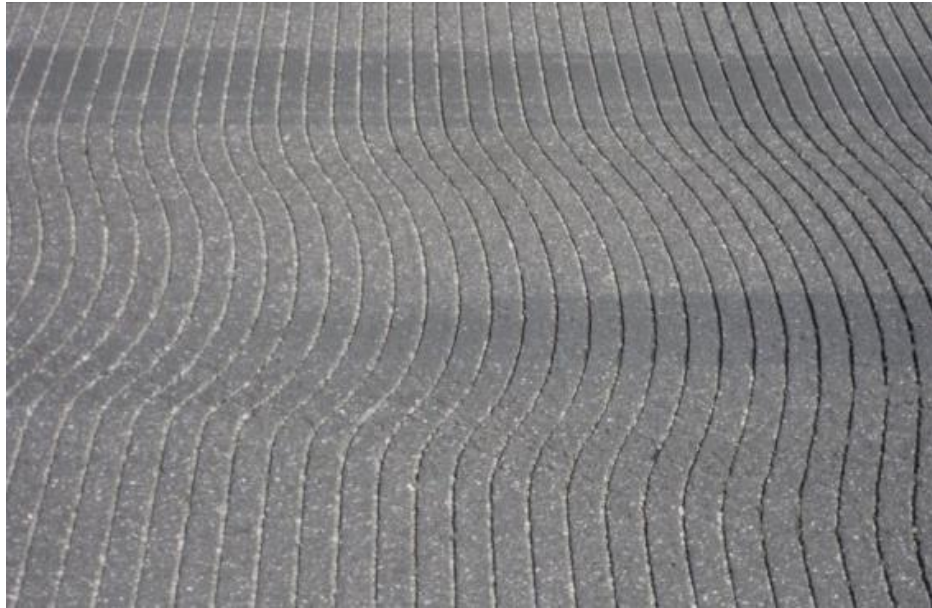
Figure 1: Example of typical horizontal shear creep failure
