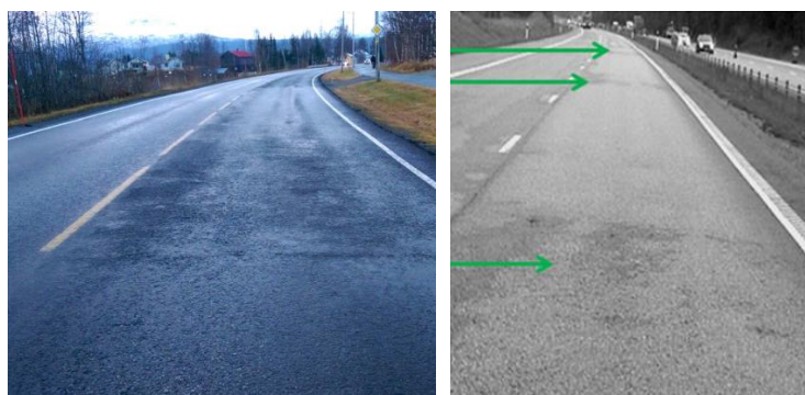
Figure 17: Cold asphalt results in defects in the asphalt pavement (Photo: Geir Johnsen, NPRA)
