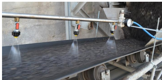
Figure 3: Spraying system installed over the RA belt
