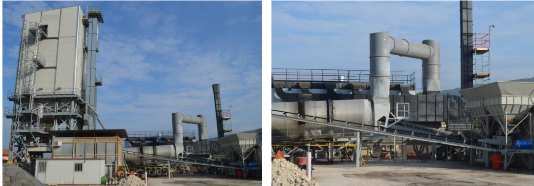
Figure 2: Overview of the mix-plant, with the belts that convey the RA before and after the drier
