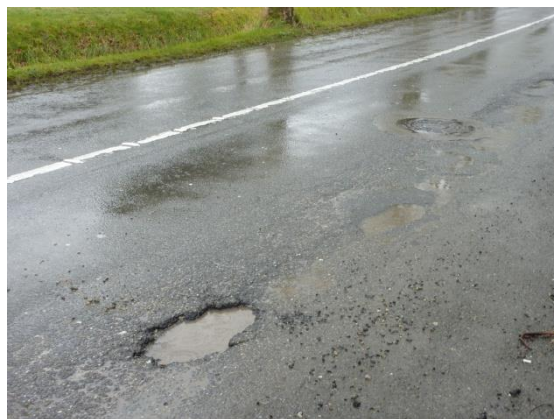
Figure 1 – Road with pothole
