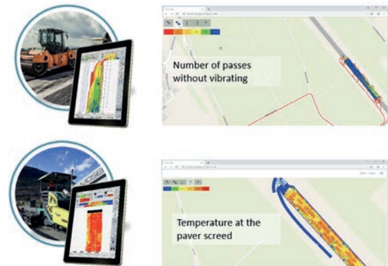
Figure 8: GPS based measurement and visualisation and reports of the paving and compaction process.
