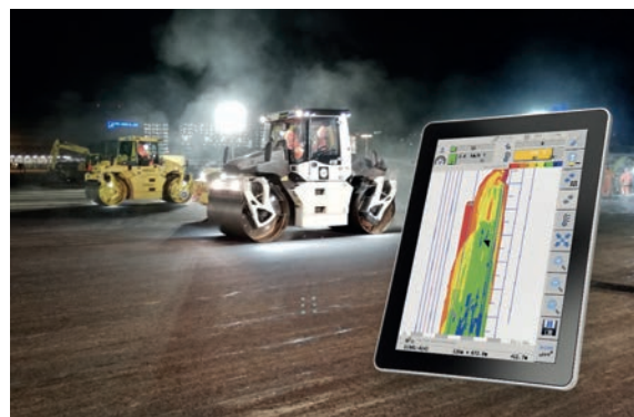
Figure 7: Digital compaction control at ARGE Midnightforce – Renovation of runway 10/28 at Zurich airport by Walo Bertschinger (CH) and Implenia (CH).
