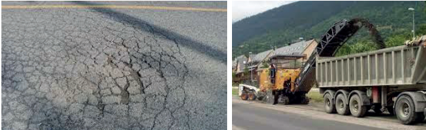
Photograph 4: Deteriorated section and recovery of the milled bituminous mix
