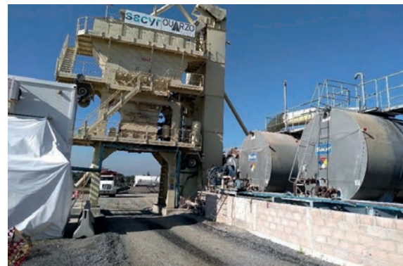
Photograph 1: Asphalt plant for the production of hot bituminous mix
