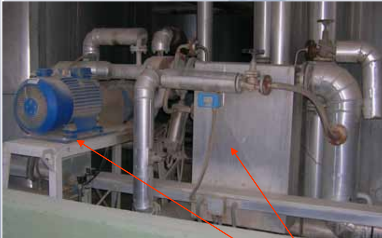
“Hard” bitumen feeding pump + massic metering
