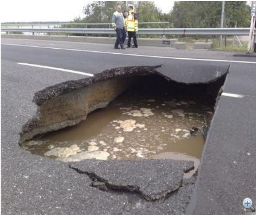
Figure 2: Collapsed section of motorway M1 in 2009 (Hungary)
