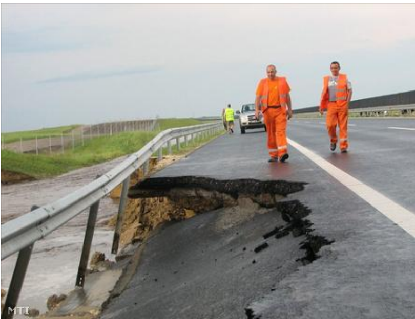
Figure 3: Collapsed paved shoulder in motorway M6 in 2010 (Hungary)
