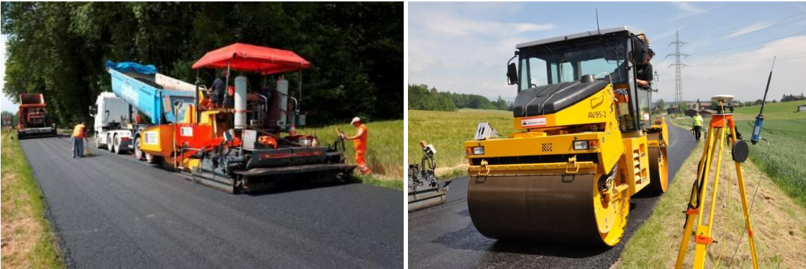
Figure 12: Two pavers and roller compactors, e.g. AV 95-2 ACE (with GPS based compaction control ACEplus).
