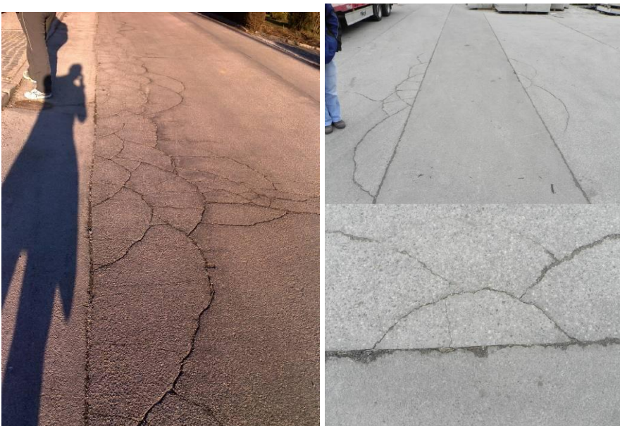
Figure 1: Semi-circular shaped cracks at the edges of the pavements (left) and excavations (right)
