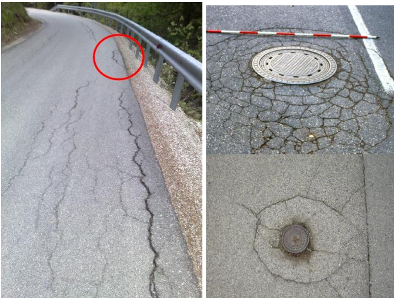
Figure 2: Longitudinal edge cracks at the edge of the pavements (left) and circular shaped cracks at the shafts (right)
