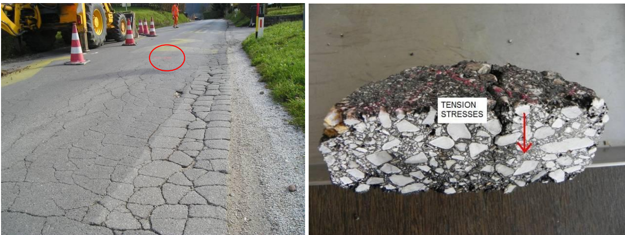
Figure 5: The location of asphalt core taken on semi-circular shaped cracks (left) and presentation of semi-circular shaped cracks propagated top to bottom through the cross section (right)
