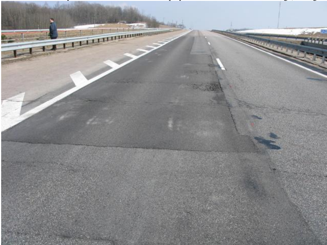
Figure. 1. Road A1 Vilnius-Kaunas-Klaipeda (216,95-220,3) km pavement structure before repair
