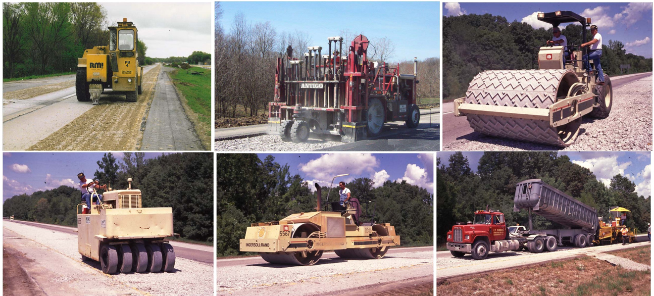
Illinois rubblizing practice: The stages of rubblizing a PCC pavement before overlaying with asphalt, both of the pavement breakers have been proved to be effective
