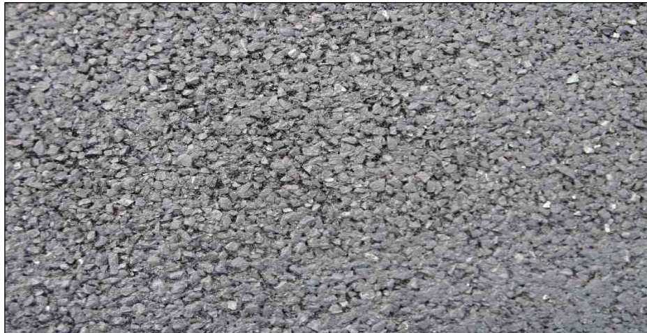
Figure 19(c) : Modified Semi-Open Graded Asphalt Friction Layer Trial (Many Surface Voids and Course Surface Texture)
