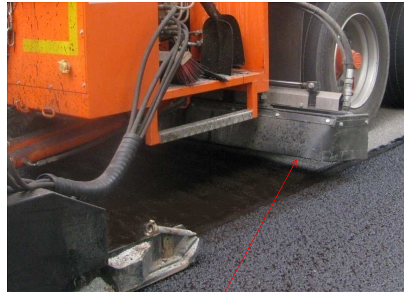
Tack-coating spraybar is installed behind the rear axle and directly in front of the micro spreader box!
