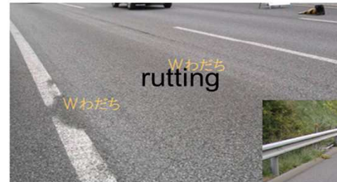
Severe pavement distresses in Expressways
