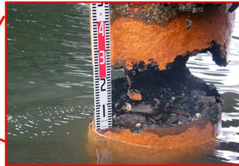
Severe corrosion of bridge pier Miharashi-bridge(Yokohama) Constructed about 40 years ago
