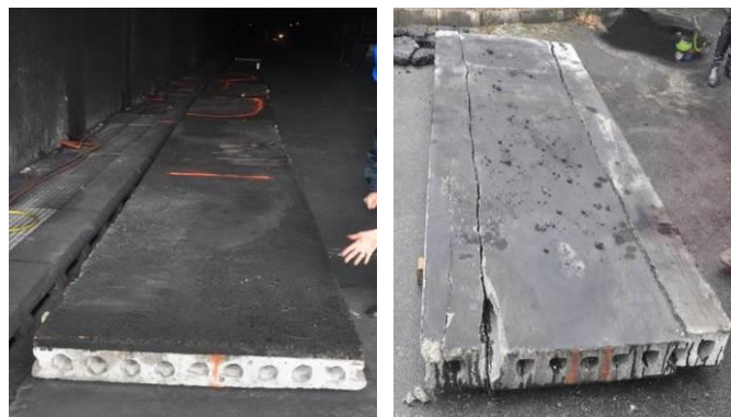
Figure 17: Surface appearance of the bituminous mixing plate containing flame retardant (left) and the concrete plate (right).
