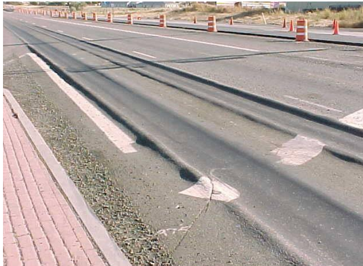
Figure 1. High severity asphalt rutting on highway
