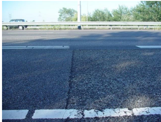
Figure 1: A highway section showing severe raveling
