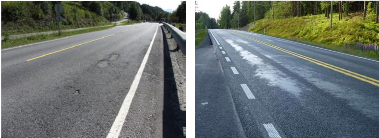
Figure 4: Typical asphalt pavement inhomogeneities (mix segregation, open vs. dense areas), these may cause both durability and poor friction problems.
