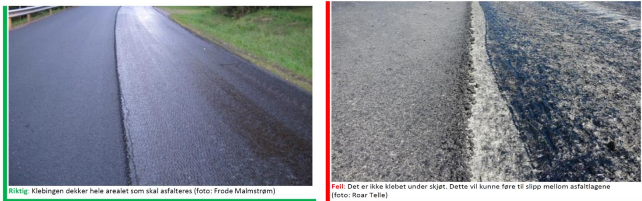
Figure 12: Example from Best practice guide; use of tack coat. Correct (left) and wrong (right) application.
