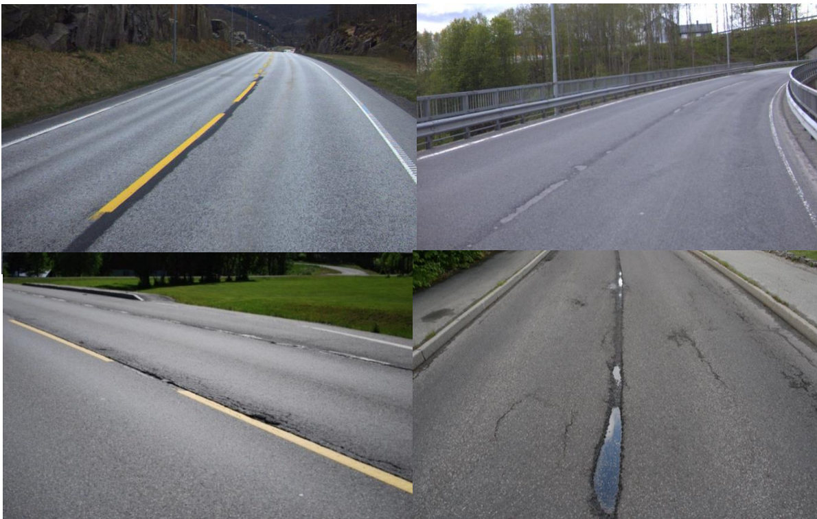
Figure 3: Typical asphalt pavement distresses due to improper execution of longitudinal joints.
