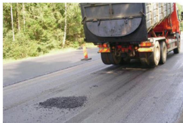
Figure 15: Examples from “Control of asphalt works”; spills from asphalt trucks shall be removed immediately, otherwise these will cause potholes.
