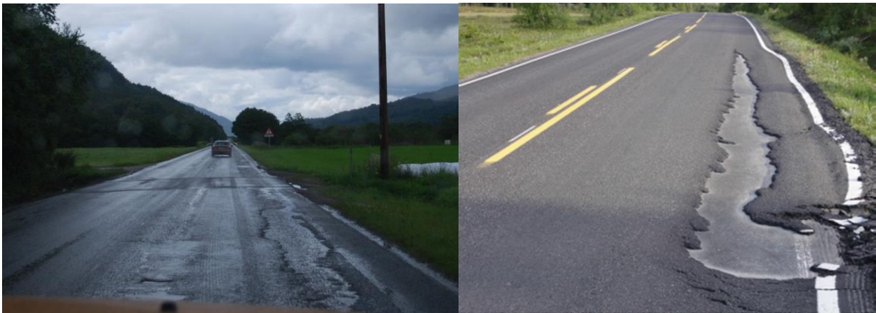
Figure 2: Typical asphalt pavement failures caused by poor interlayer bonding.
