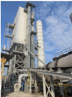
Figure 4 – Plant 2, batch plant with RA feeding
