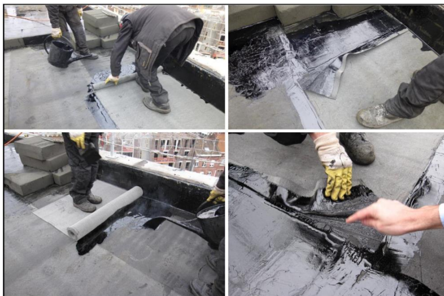
Figure 5: Bonding membrane by Bitumen B, tearing of the membrane after a tensile test.
