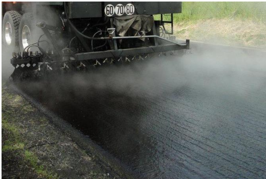
Figure 13 : uneven emulsion film during surface dressing application due to excessive viscosity of emulsion
