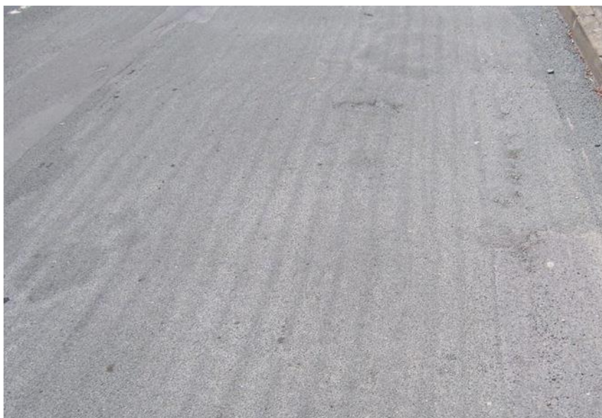
Figure 14 : surface dressing striping within months after jobsite
